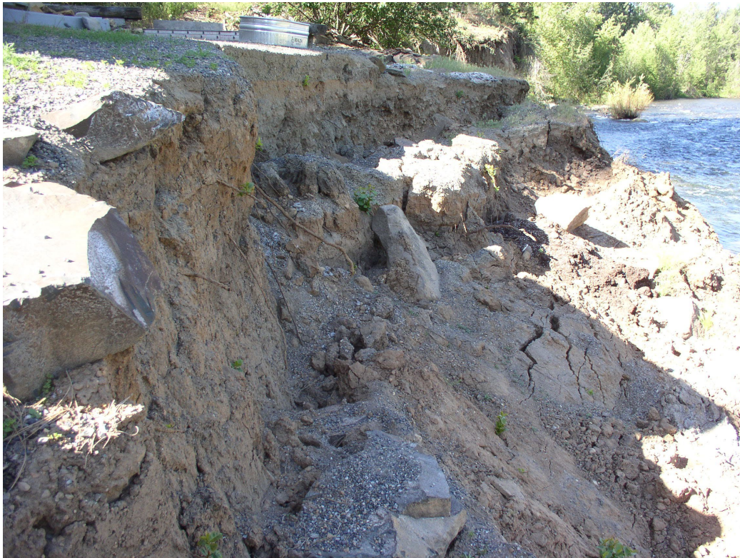
Figure 5. Image showing impacts of progressive slope failure.
