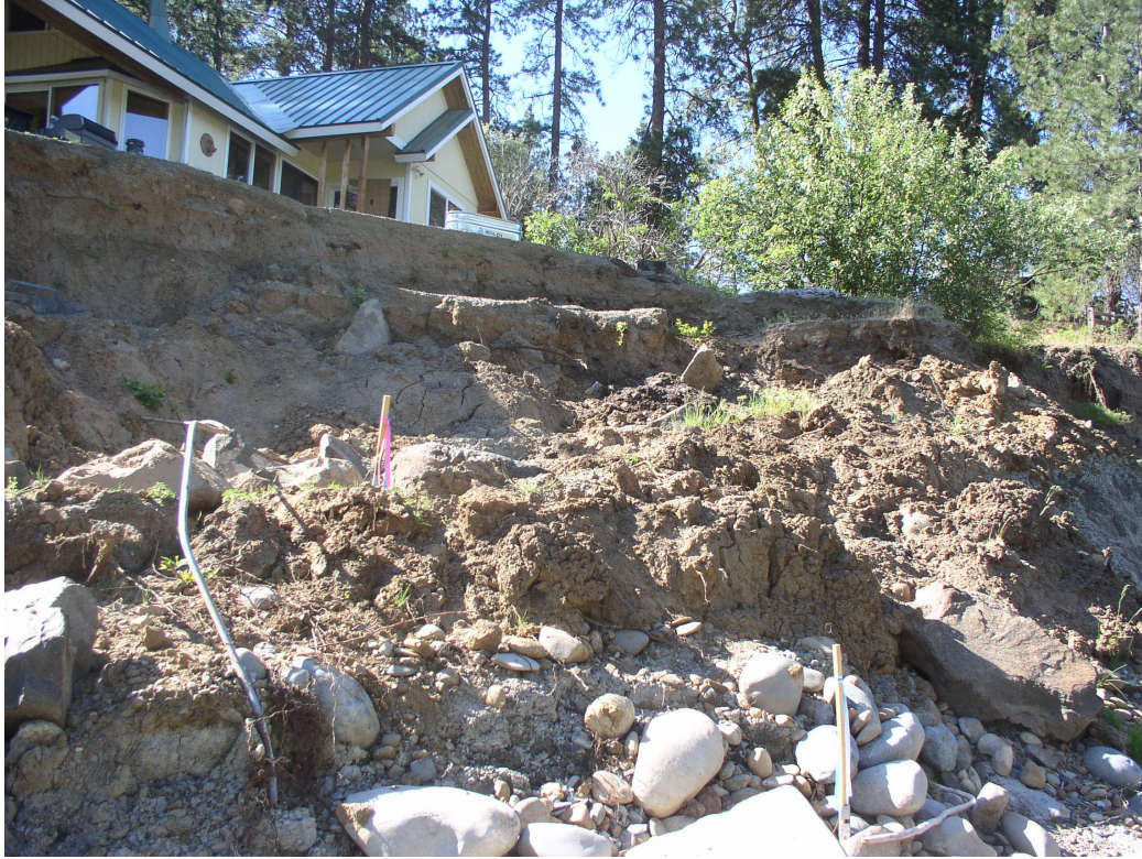
Figure 4. Image of structure at top of bank with topple, slump, and rotational failure of slope along with active cracking.
