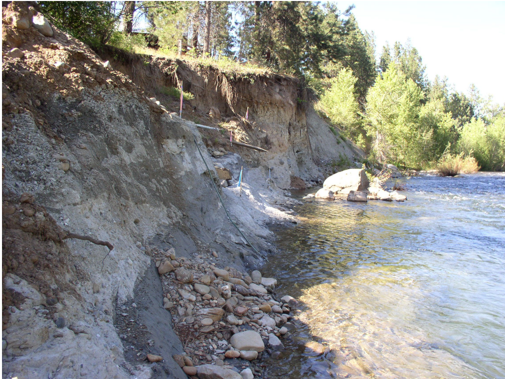
Figure 3. Near vertical streambank with cracks and wet surface from bank saturation.
